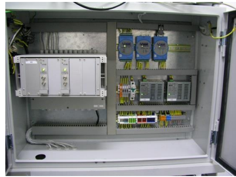
Switchboard with environmental measurement system
