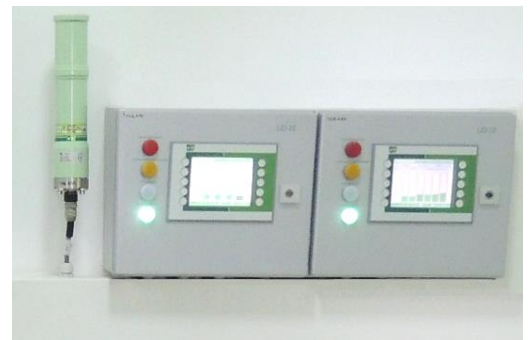
LZJ-22 Local Display Unit in the operator's workplace. On the left is the MDG-07 monitor to measure the gamma dose rate.
